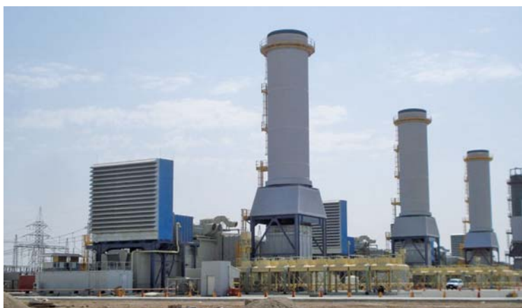
The Erbil Gas Power Plant, one of three privately built and operated plants in the Kurdistan Region, first came into service in 2008. (KRG Ministry of Electricity photo)
