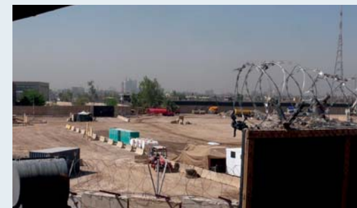
INL spent more than $100 million renovating facilities at former Forward Operating Base Shield, which was to be the main PDP basing area, before terminating construction, removing all advisors from the site, and turning the property over to the GOI.
