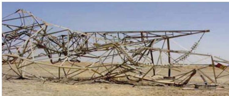
Primarily because of looting and sabotage, almost 1,000 electrical towers were destroyed and control systems were damaged, causing Baghdad and beyond to experience frequent blackouts in mid-2003. (Bechtel photo)
