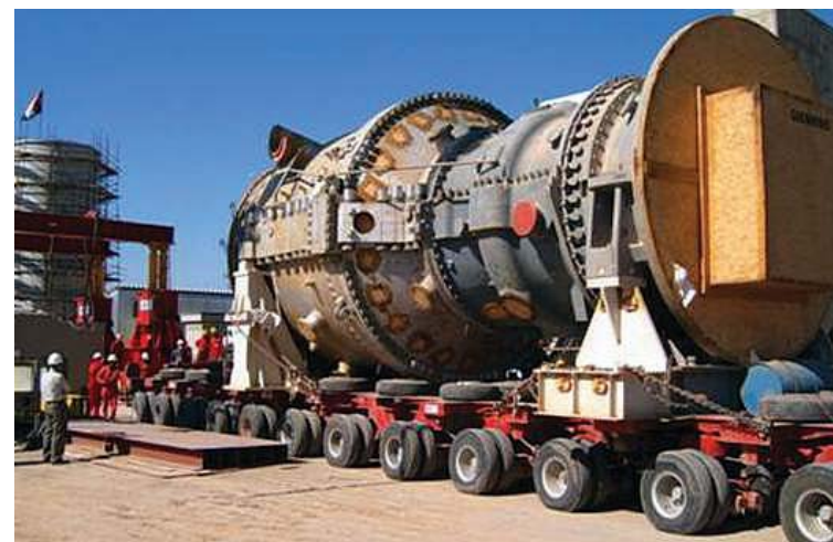
As part of a $174 million U.S.-funded project that began in August 2003, a 600-ton, 260 MW combustion turbine is delivered to a substation near Kirkuk in April 2005, after a trip through the Middle East that took more than a year. (USACE photo)
