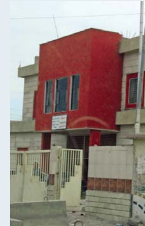
SIGIR’s inspection of the Hai Musalla Primary Healthcare Center revealed that U.S.-funded equipment was not being used because Iraqi staffs had not been trained to operate it.
