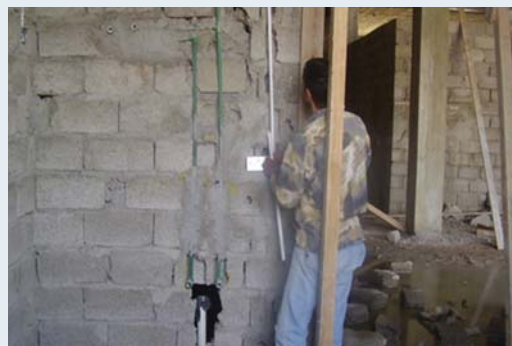
SIGIR inspects a poorly constructed block wall, one of many deficiencies that SIGIR identified at PHCs throughout the country.
