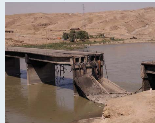
Coalition bombing damaged al-Fatah Bridge in 2003.
